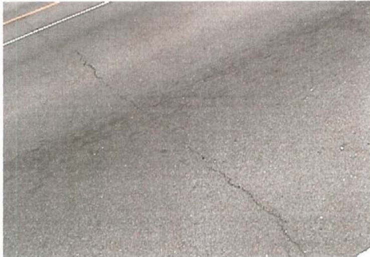
SM. CRACK AT APPROACH #1
