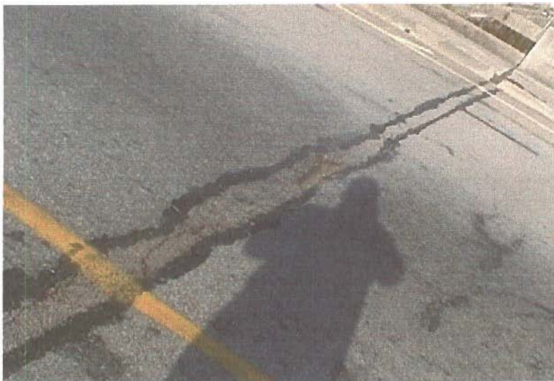
VOID IN SEAL IN EXPANSION JOINT AT #2 END
