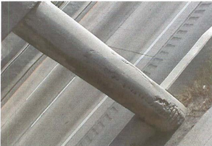
BENT #1, COLUMN F, LARGE DELAM WITH REBAR EXPOSED
