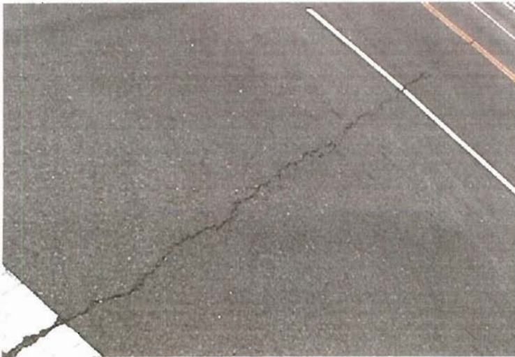
SM. CRACK AT APPROACH #2
