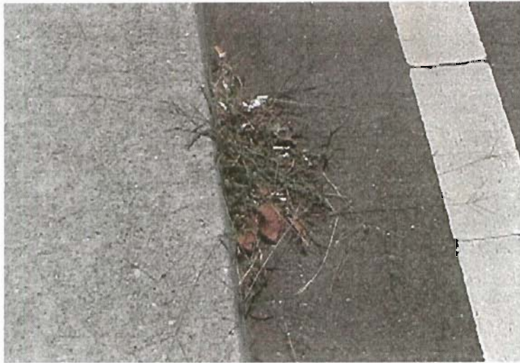
VEG. IN DRAINS
