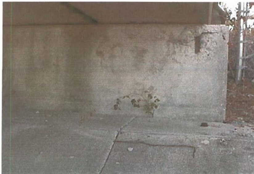
ABUTMENT #1, LEFT SIDE, LARGE DELAM AREA
