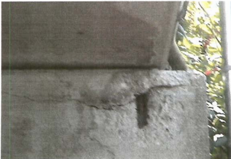
SPALL W/ REBAR EXP. #1 ABUT
