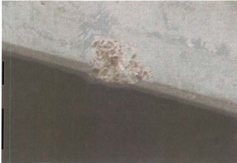
ABUTMENT #1, LEFT SIDE, LARGE DELAM AREA
