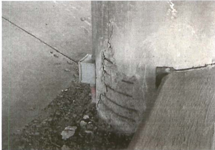
SPALL W/ REBAR EXP. BENT #1 COL
