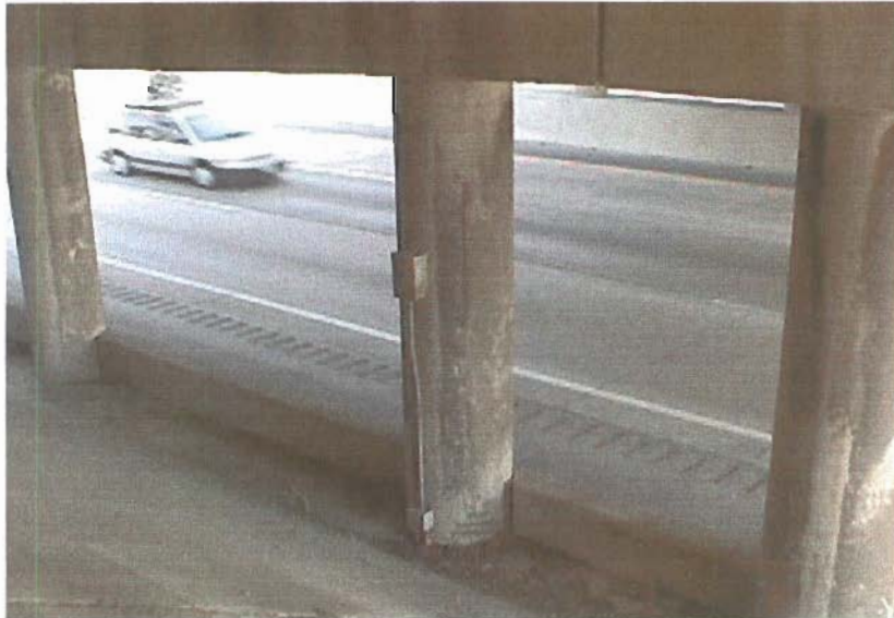
BENT #1, COLUMN C, LARGE DELAM WITH REBAR EXPOSED
