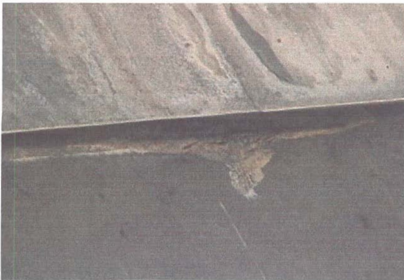
SPAN #3 BEAM A, SPALL W/ STRANS EXPOSED
