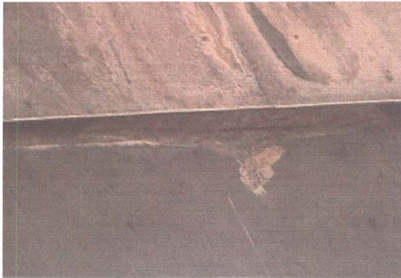
SPAN #3 BEAM A, LARGE SPALL W/ STRANS EXPOSED
